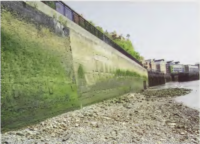
FIGURE 7. Near-vertical river wall at Wapping; the brick wall in the foreground is covered by green algae while the concrete wall in the background has a less-extensive cover, May 2012.
